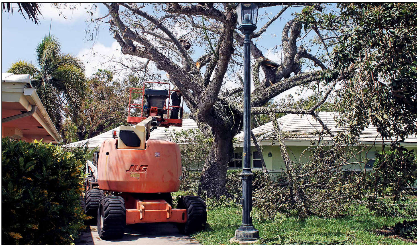
JKV Grounds crews were clearing tree damage the day after Hurricane Irma hit the Village in 2017.
