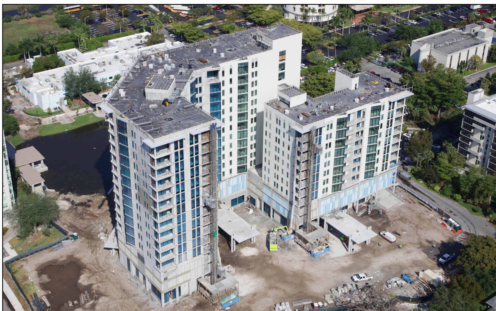
The 15-story Vue and 11-story Terrace have completed the air-conditioning system installation and are now undergoing interior finishing.
