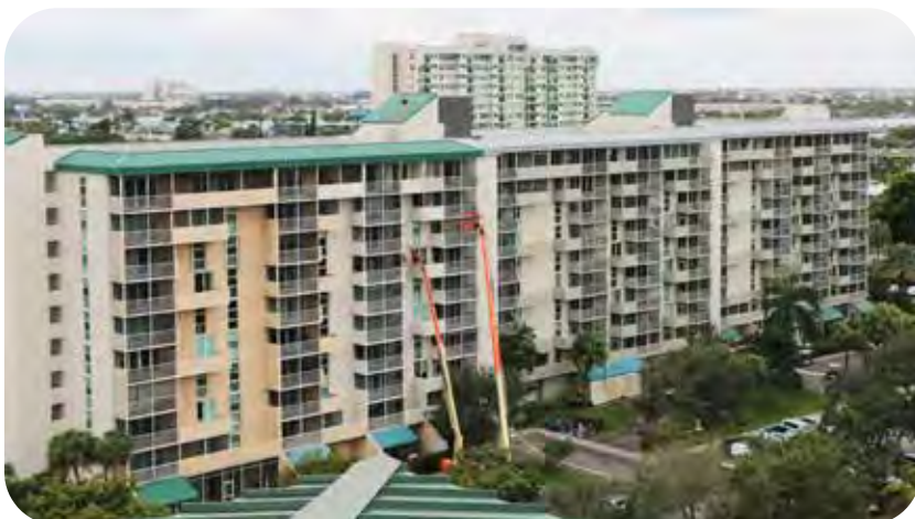
As seen from the Heritage Tower rooftop, the exterior of Village Towers is getting a facelift, including the installation of impact windows and sliding glass doors, waterproofing and painting.
