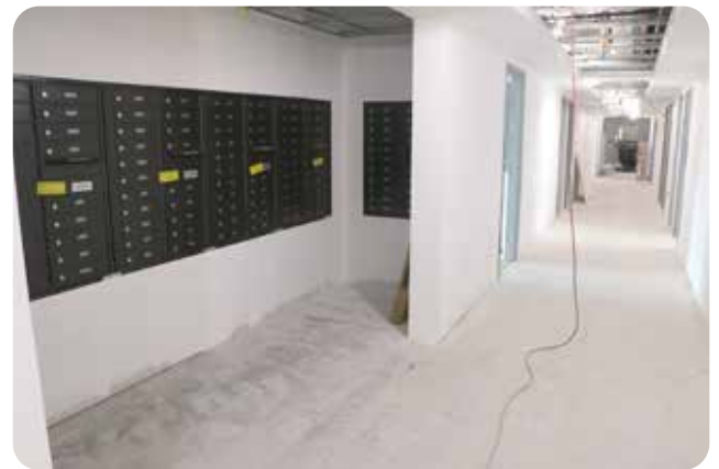
The Cassels Tower first-floor conversion of Administrative offices into apartments is progressing well. This view looks west, with new Resident mailboxes on the left.
