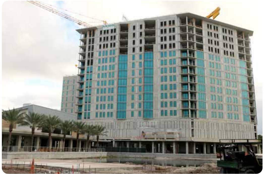
The shell of Westlake—The Vue and The Terrace—has been completed. This view is looking east with the Pavilion on the left and expanded Rex Foster Lake in the center.
