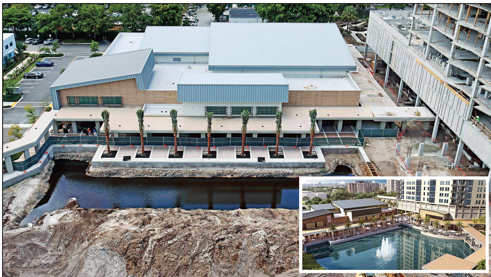
Rex Foster Lake, in front of the newly opened Pavilion, is currently being excavated. When completed, it will connect with Lake Maggie to offer waterviews in The Vue and Terrace apartment buildings now under construction.
