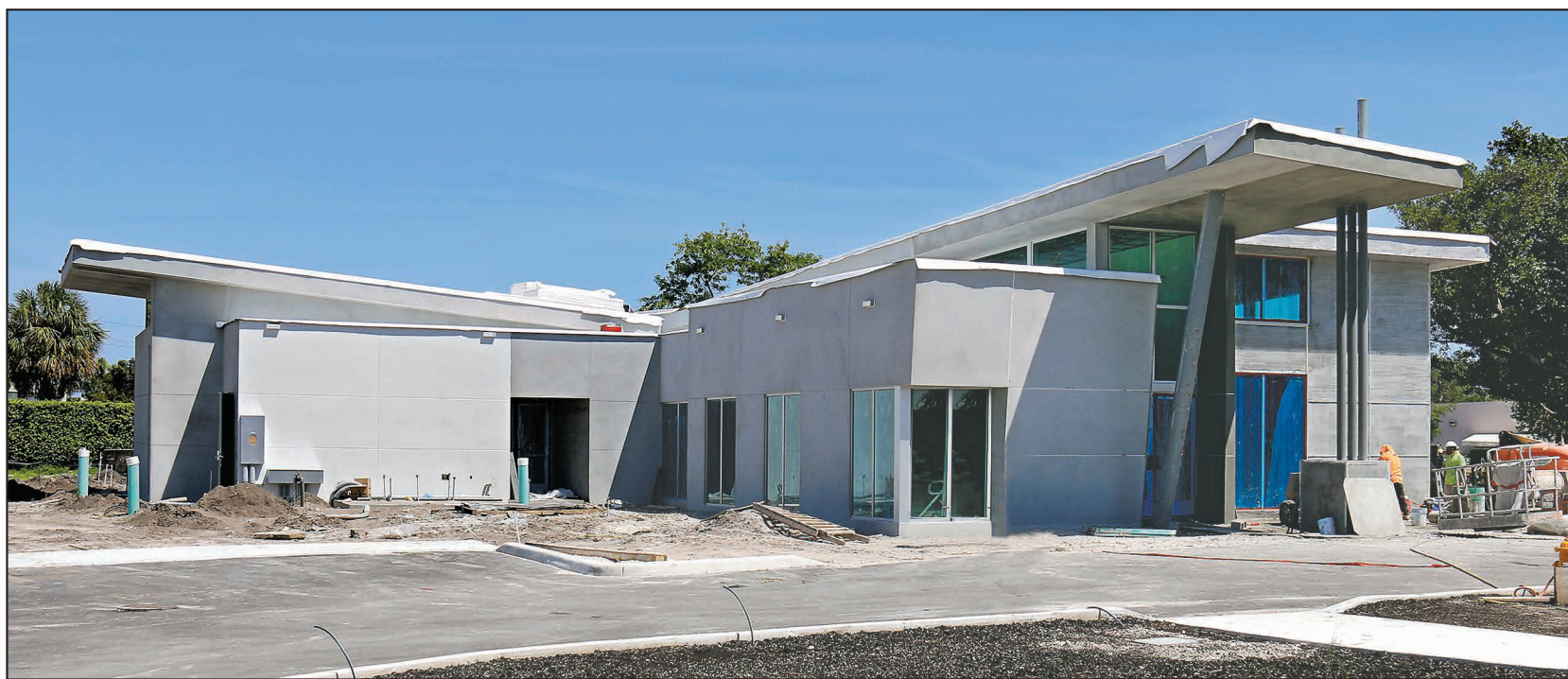
The Welcome and Innovation Center at John Knox Village finalizes construction for a projected opening this month.
