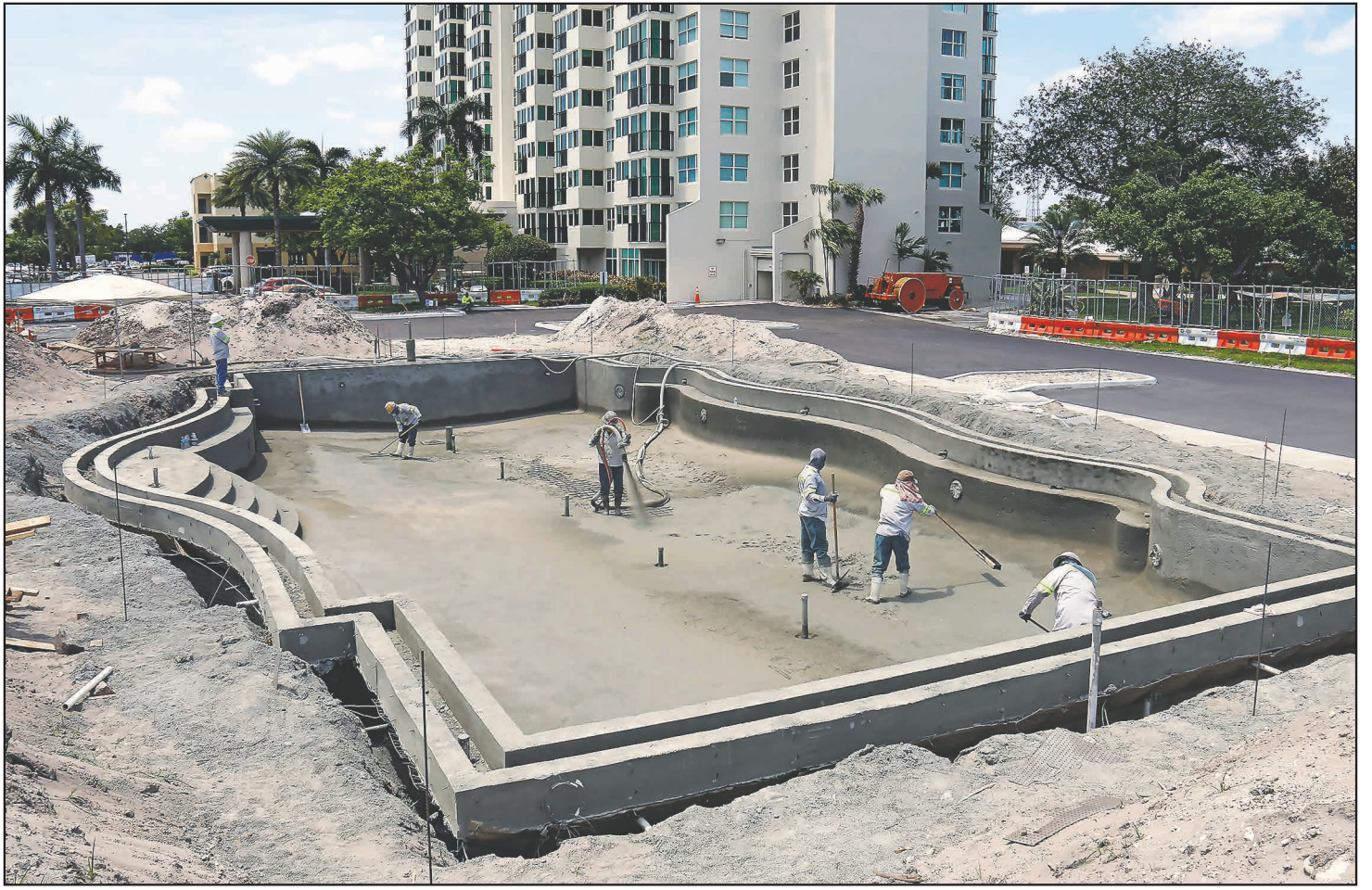
The large resort-style lap pool is under construction at John Knox Village.
