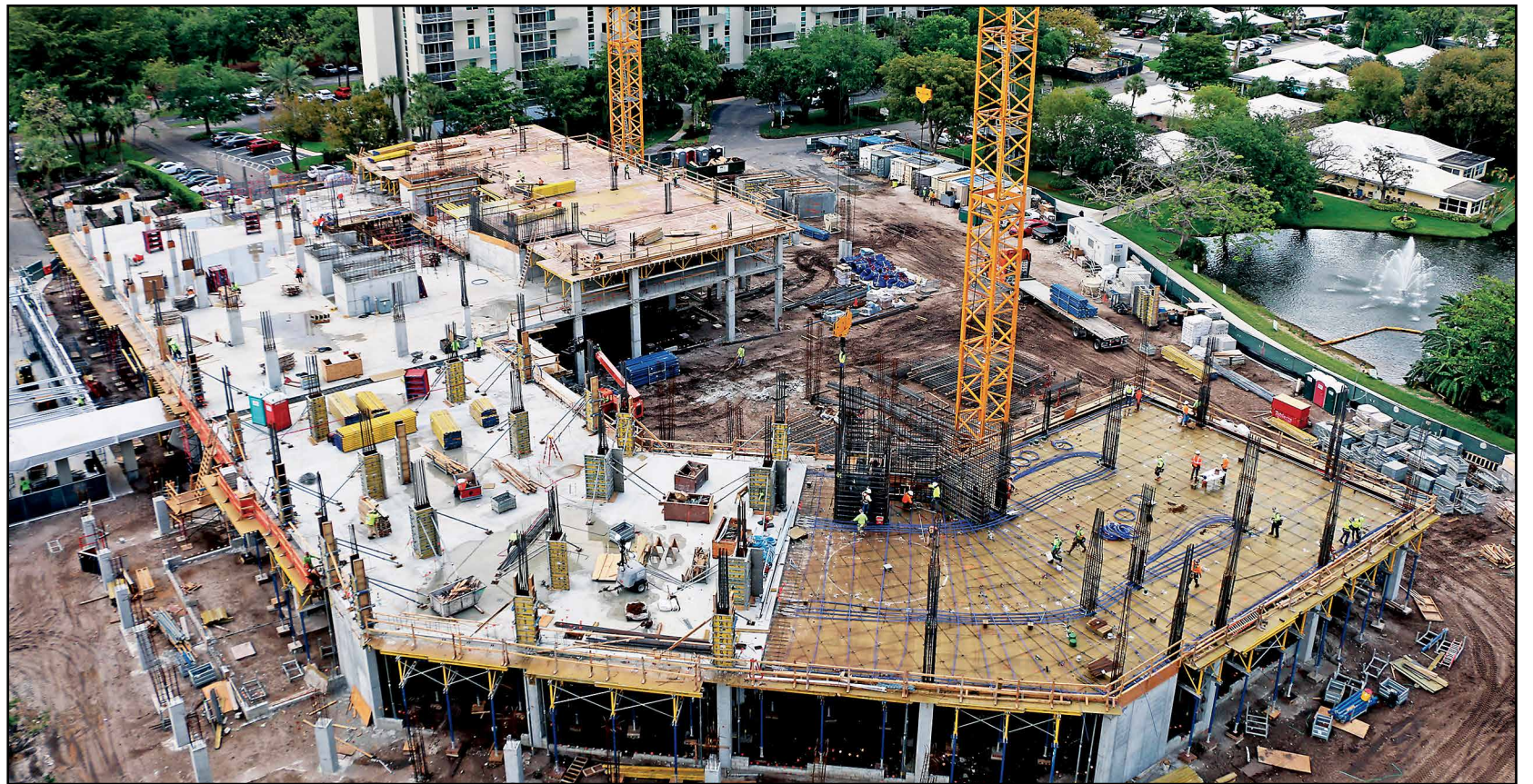
The twin towers of The Vue and The Terrace at Westlake are spiring upward. When completed, the Vue will top at 15 stories and The Terrace at 11 stories. A total of 146 new apartment homes will overlook the reconfigured Lake Maggie and Rex Foster Lake.
