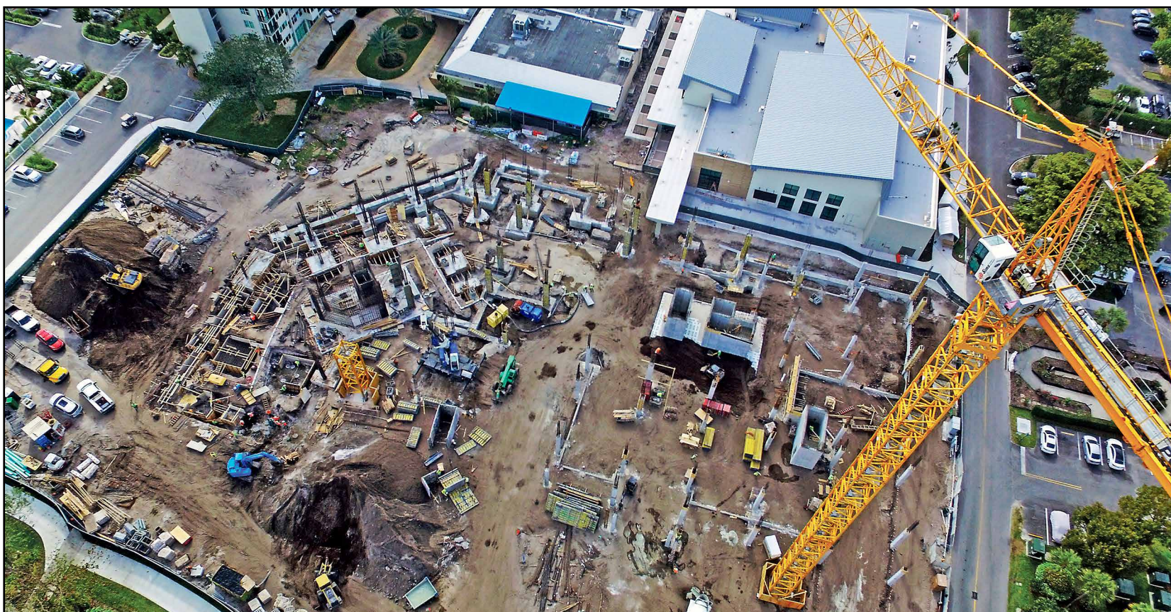
The JKV drone recently captured construction on the twin towers. The Vue and The Terrace at Westlake. The nearly completed Pavilion with its two restaurants and 400-seat Performing Arts Center, is at upper right.
