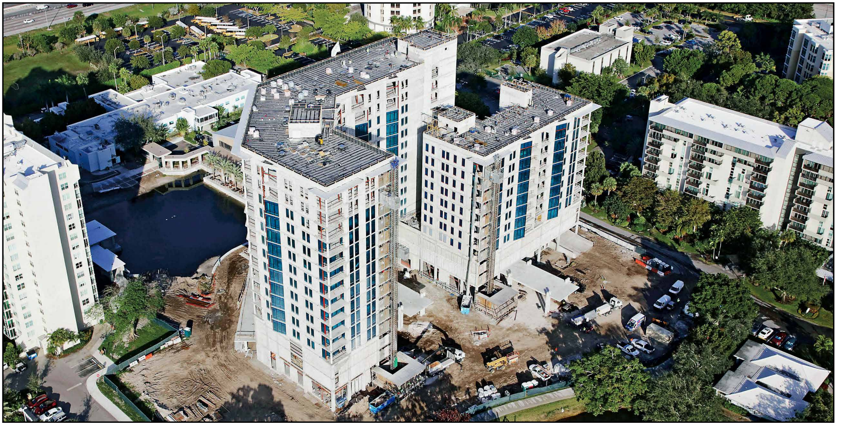
The pair of construction cranes that helped build the shells of The Vue (left) and The Terrace have been removed.
